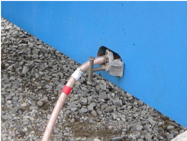
Fig. 2 Incorrect Clamp Used for Application
